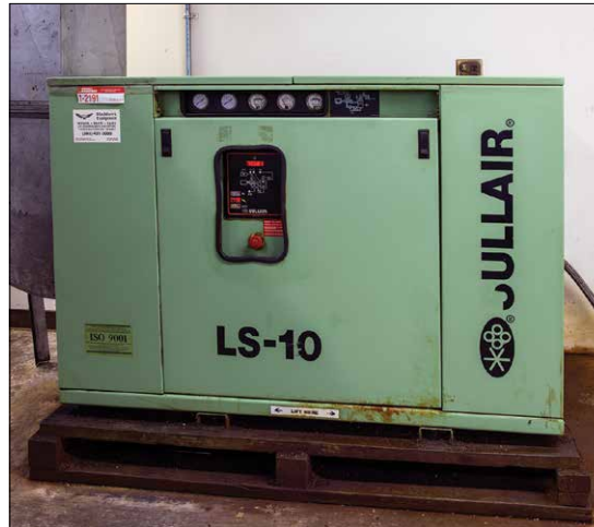
Sullair LS-10 25 HP Rotary Screw Air Compressor
