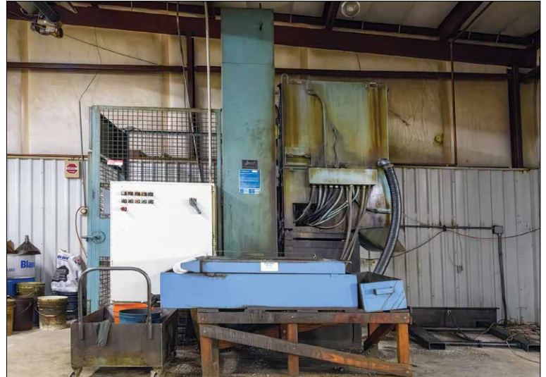
Steimel Chip Reclamation System
