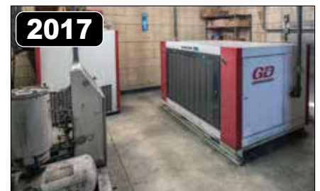
Gardner Denver Air Compressor & Dryer
